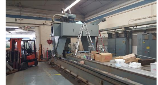
High speed core router retrofit
